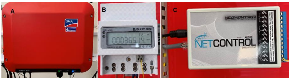
Fig.3. Grid inverter and electricity meter device: A – Grid inverter Sunny Boy 1.5; B – Electricity meter EJS 212 D20; C – Pulse counter NET Control.
